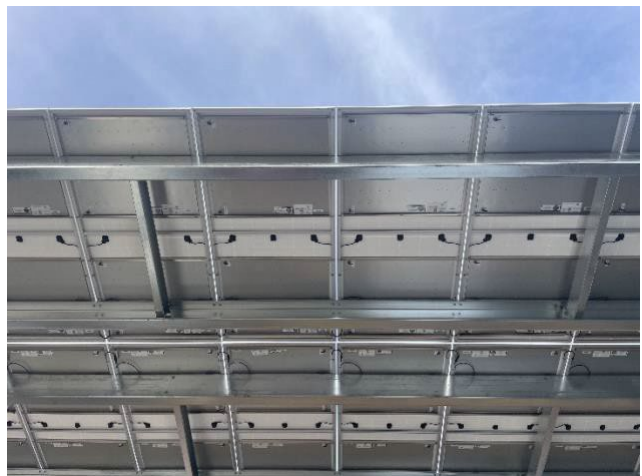
PV thermal heat collectors are placed beneath the solar PV arrays to provide thermal energy for the building and pool.
