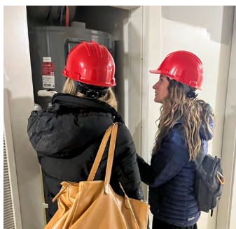
Jackie Slocombe of Mercy Housing and Lauren Westmoreland of Stewards of Affordable Housing for the Future examine a semi-centralized hot water system.
