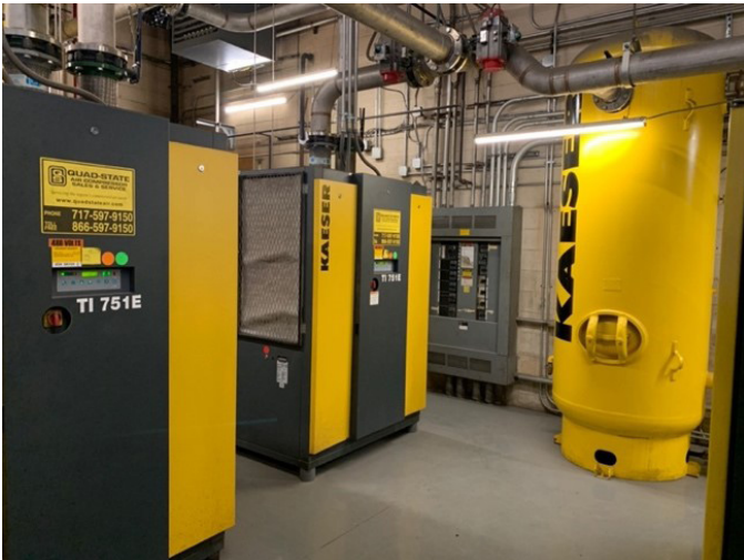
The new compressor room was the largest project that was completed at 1 JLG Drive. Courtesy of JLG.
